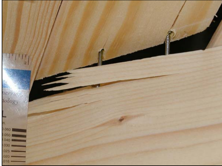
Figure 4.23 Joist splitting at point of nailing (DDR = 1.5 %)
