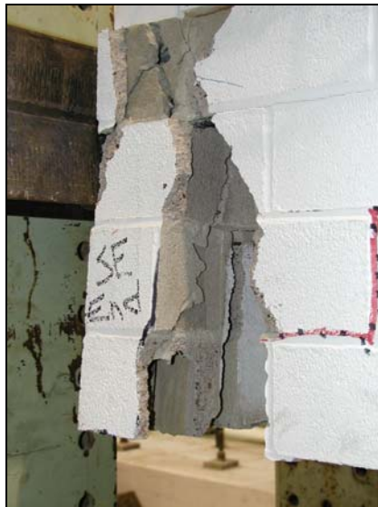
Figure 4.27 Deterioration of masonry chord at maximum diaphragm drift ratio (DDR = 2.3 %, southeast corner)
