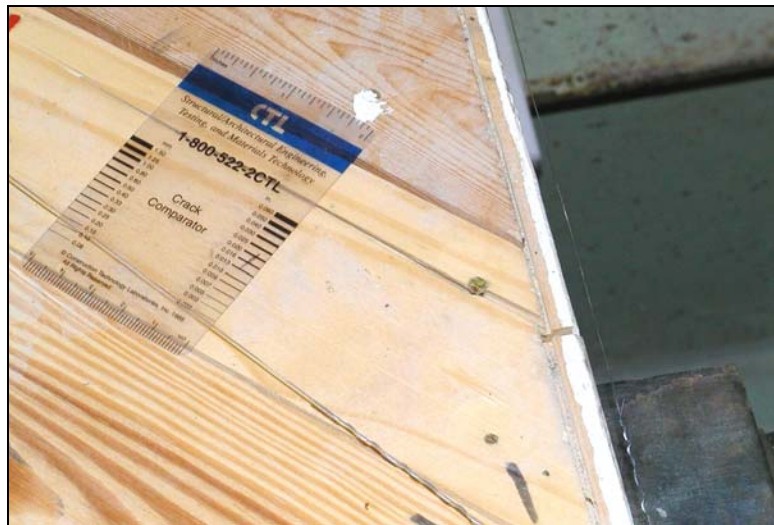
Figure 4.14 Longitudinal splitting at point of nailing (DDR = 0.3 %, east side of south quarter)
