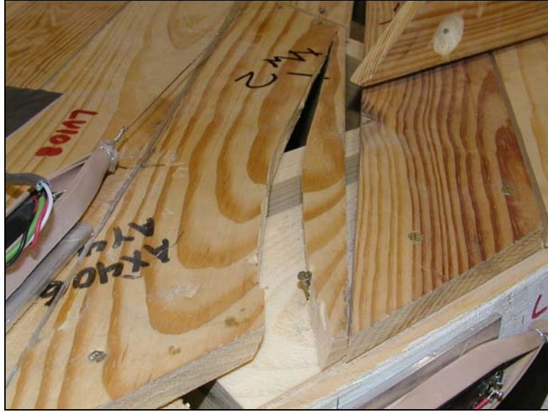
Figure 4.28 Longitudinal splitting of sheathing board at point of nailing at maximum diaphragm drift ratio (DDR = 2.3 %, northwest corner)
