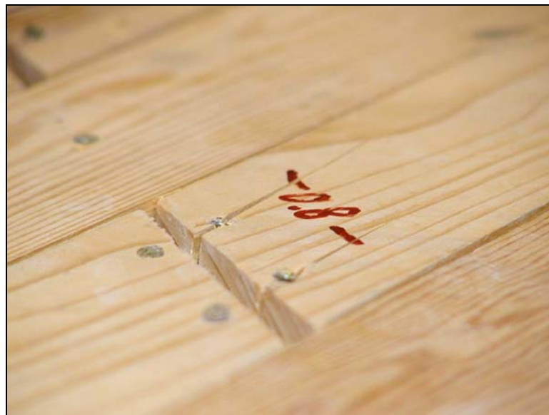
Figure 4.16 Longitudinal splitting of sheathing board at point of nailing and spreading of butt splices (DDR = 0.6 %)
