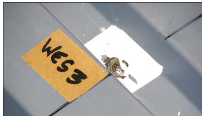
Figure 4.33 Flaking of Hydrostone® weld coating
