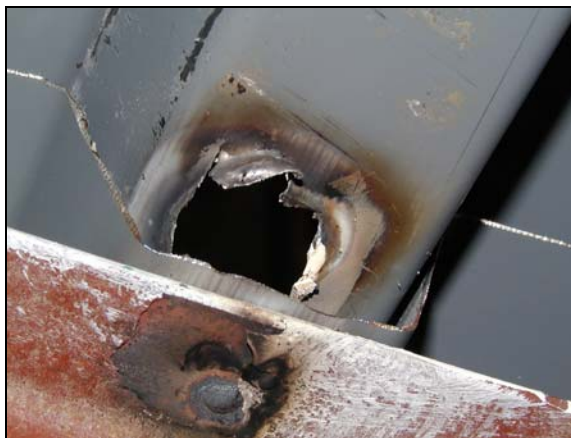
Figure 4.39 Example of weld “tear out” at joist-to-weld interface
